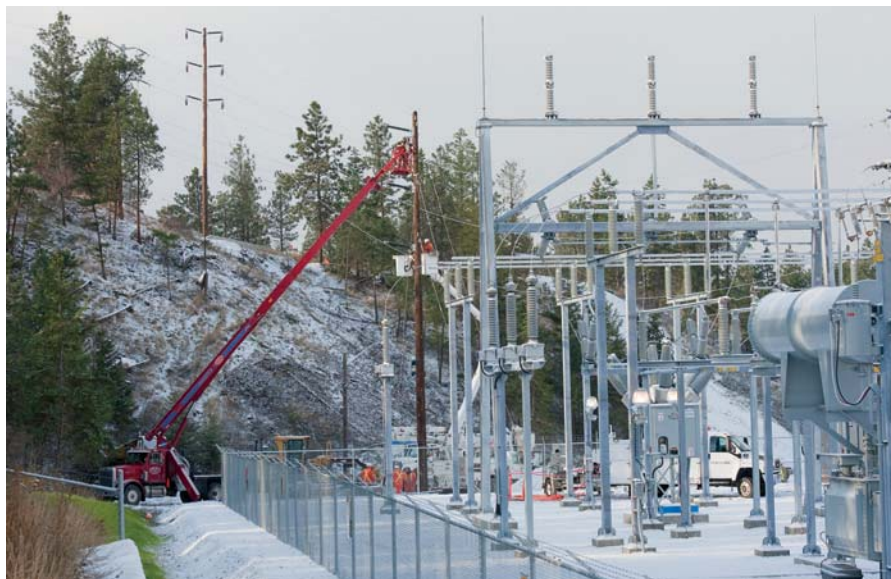
Capital work in 2010 included construction of the Benvoulin substation in Kelowna, British Columbia.
